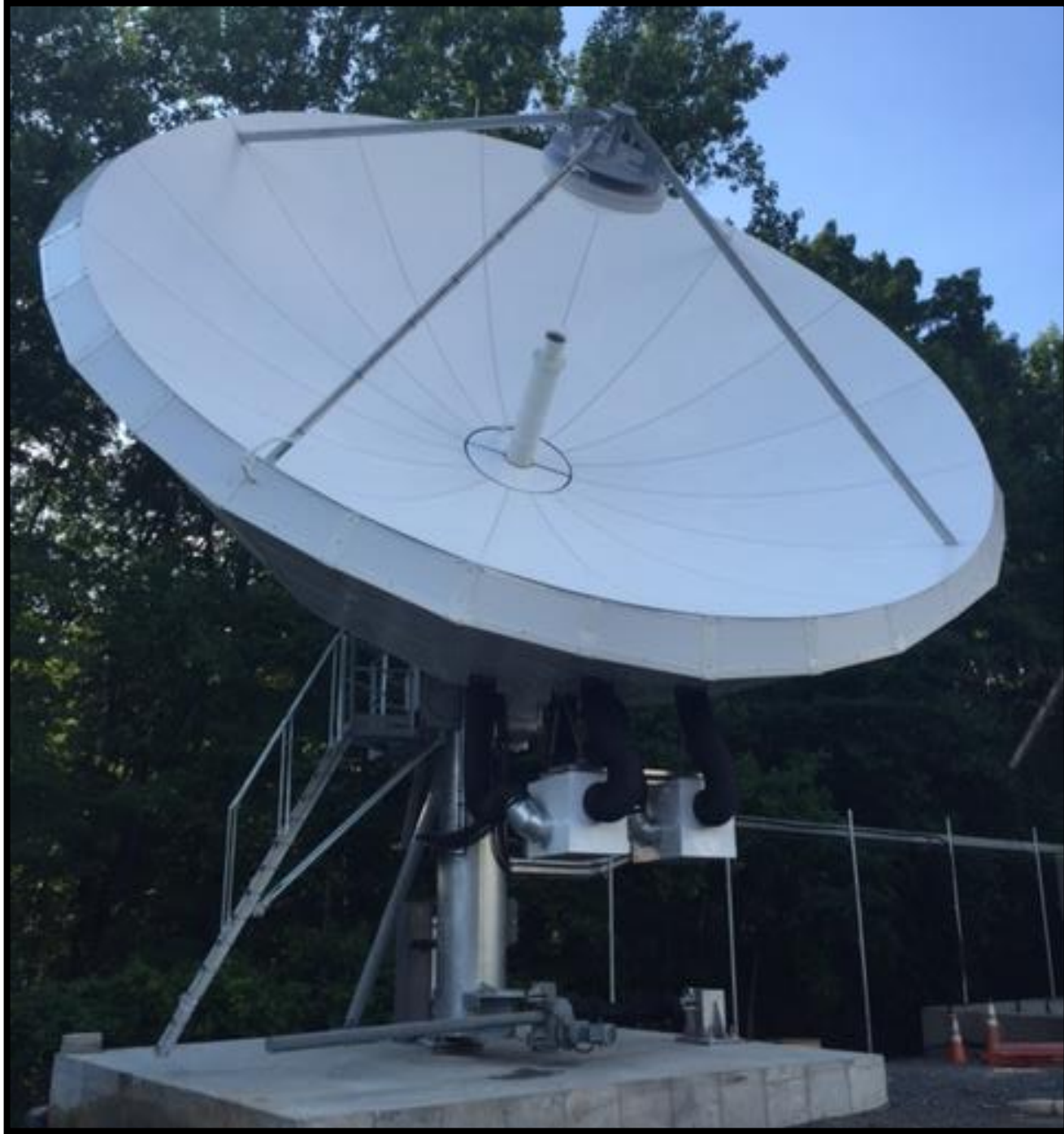
9.0-Mtr Ku-band Lo-PIM Antenna Holmdel, N.J. Note: Azimuth Jack Attached to the pedestal
